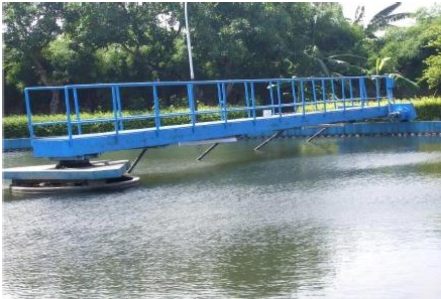
Gambar 8. Bak Pengendap II ( Secondary Clarifier )
